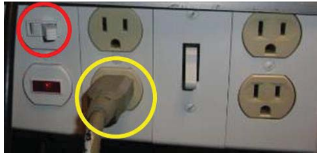
FIG. C.5. ESD power supply switch (outlined in red). This switch controls the bank of plugs to the right of it. In this image the current position is “on,” turned to the right and the CPS power supply cord is outlined in yellow. The red light (under the switch) indicates that the power supply is on and the user should take caution.
